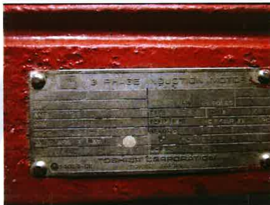
Pompa Utama ( Electric Pump )
