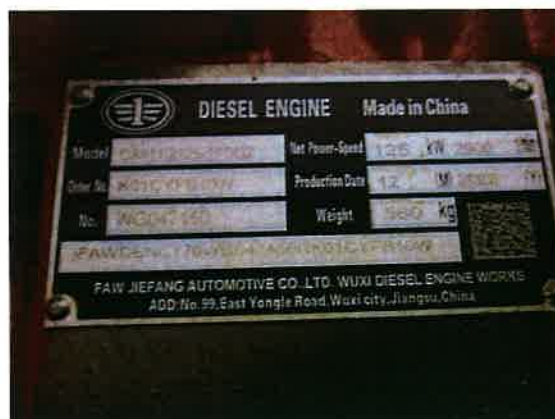
Pompa Cadangan ( Diesel Pump )
