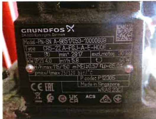
Motor Pompa Pacu ( Jockey Pump )
